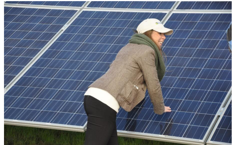
Example of touch safe technology at Keystone Solar, PA
