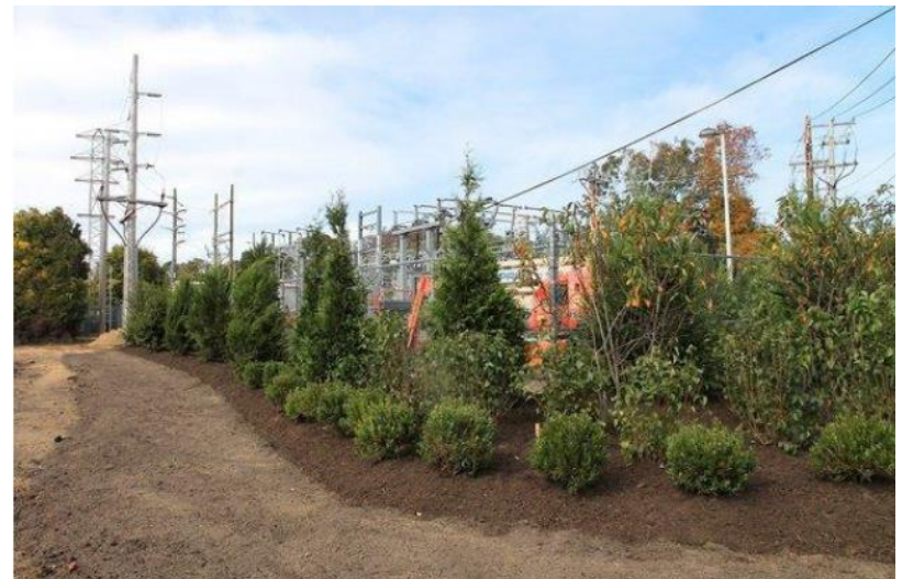
Example of substation with vegetative screening
