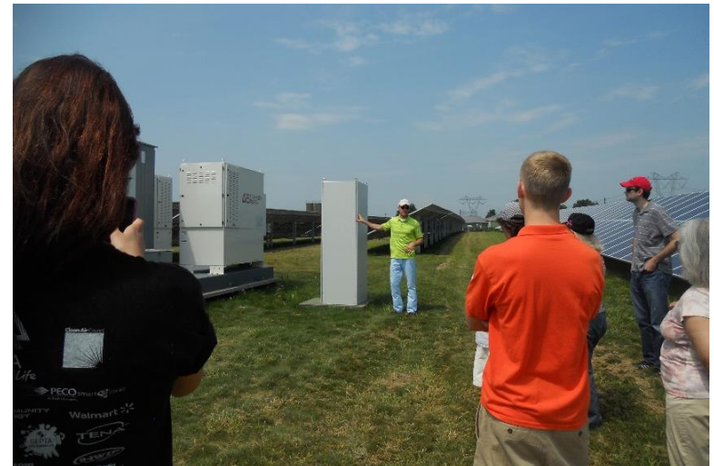
Example of Solar Inverter at Keystone Solar, PA
