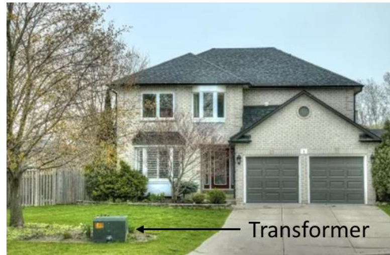
Example of residential transformer box for reference
