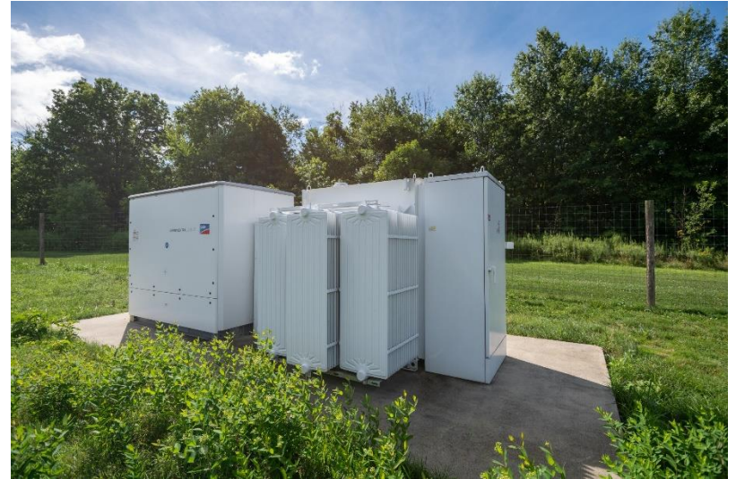
Example of solar transformer at Elizabethtown College Solar, PA
