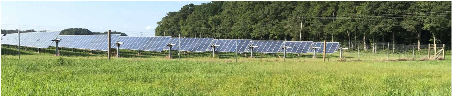
Example of agricultural style fencing at Amazon Solar, VA
