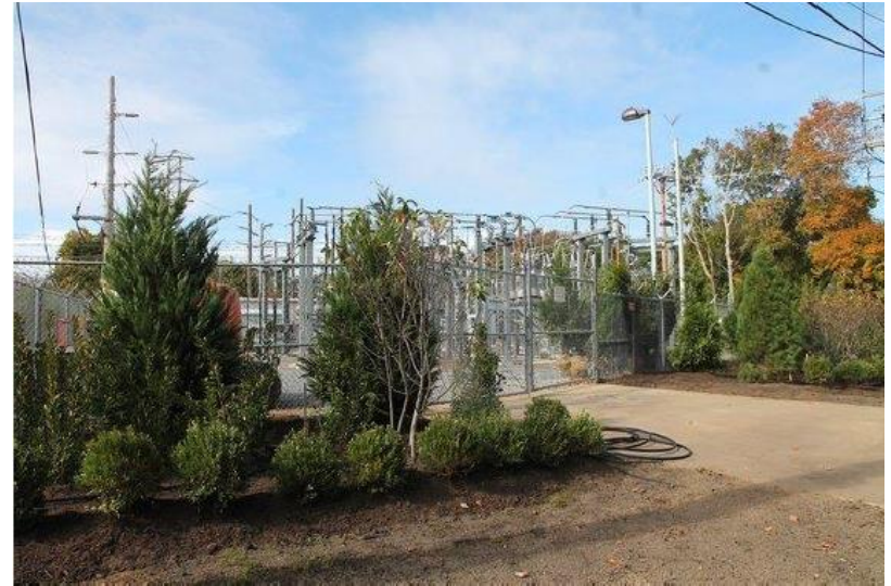
Example of substation with vegetative screening
